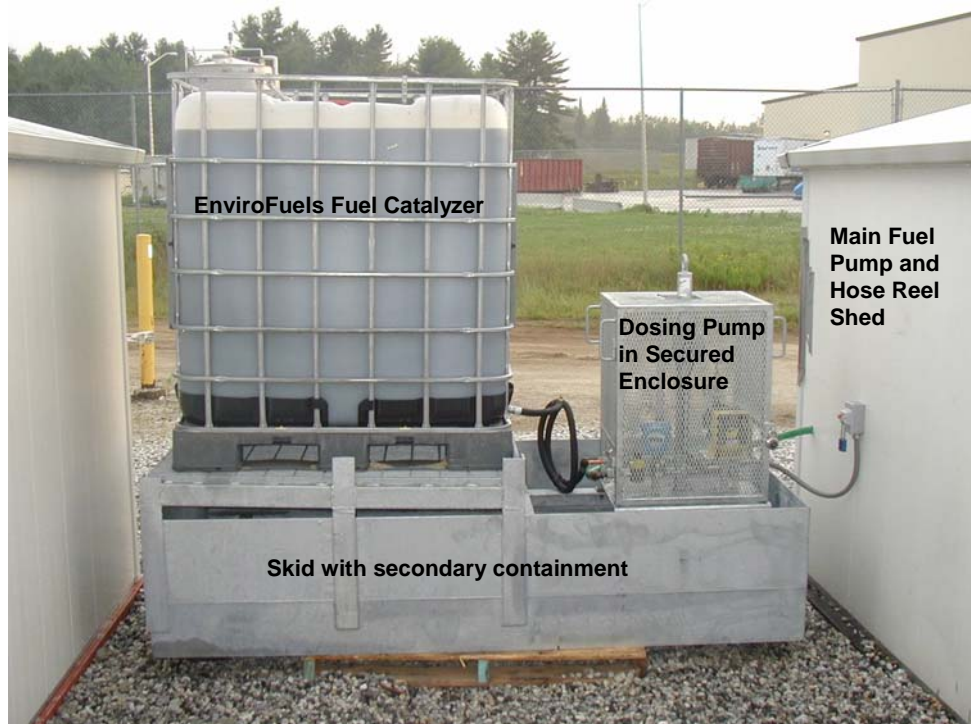
Figure 1-2. EnviroFuels Tote, Dosing Pump, and Skid
