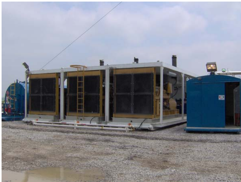
Figure 3: Three Caterpillar D399 Engines on Rig 412
